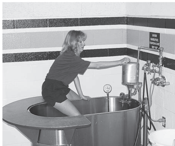
Figure 5–35 When a therapeutic device is not properly grounded, there is danger of electrical shock. This is a major problem in a whirlpool.
