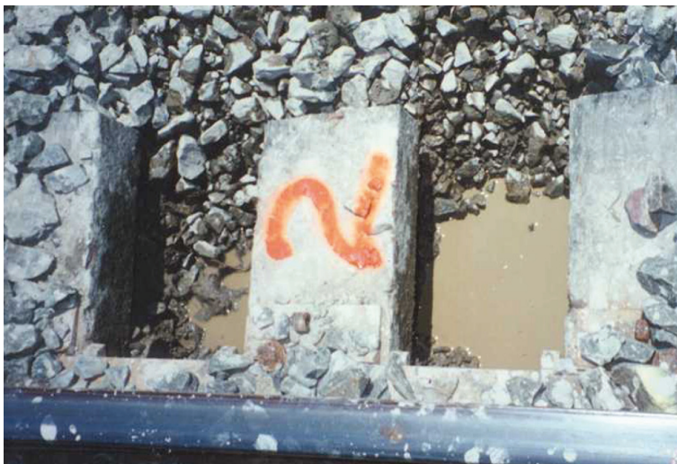
Figure 1.6 Ponding water in the load bearing ballast along a Sydney metropolitan line in Australia.
