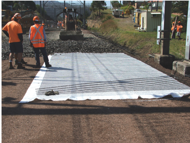
Figure C1 Laying the Geogrid over non-woven geotextile to form a geocomposite layer in fully instrumented rail track at Bulli town north of Wollongong City, New South Wales.
