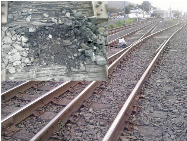
Figure C10 Pulverization of ballast plus coal fouling observed near v-crossing close to Thirroul, New South Wales.
