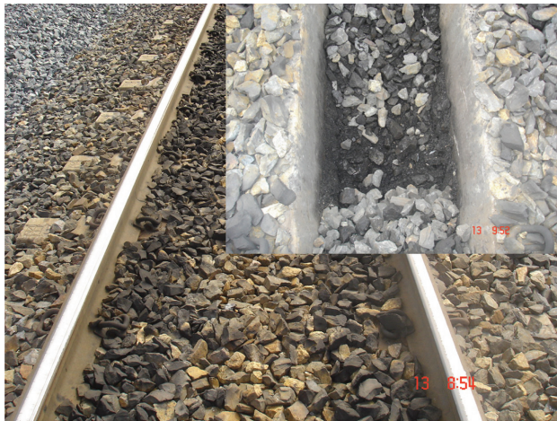
Figure C8 Migration of coal fines towards bottom of the ballast bed due to vibration and rainwater infiltration, leaving the surface ballast relatively clean – a site near Rockhampton.
