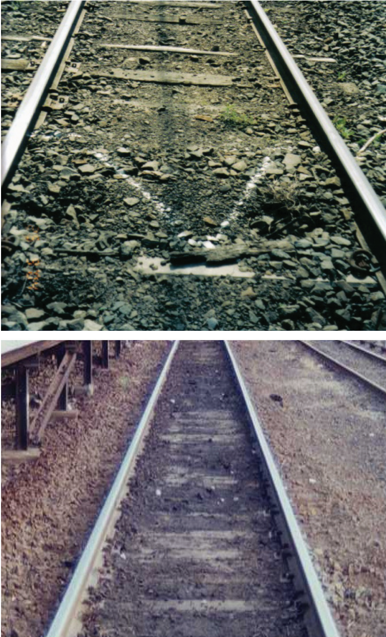
Figure 1.1 Degradation and fouling of ballast in track in New South Wales Australia.
