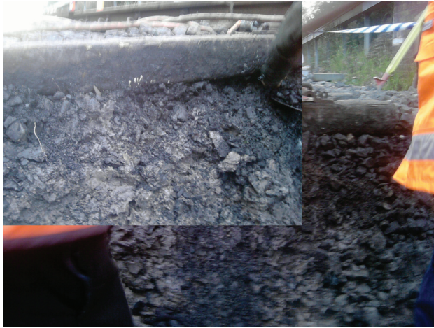
Figure C9 Coal and clay sediments fouling the ballast beneath the sleeper at a site in Thirroul, south of Sydney, observed during track maintenance.
