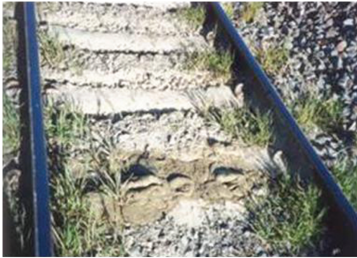
Figure 1.8 Dried slurry deposited around the sleepers.
