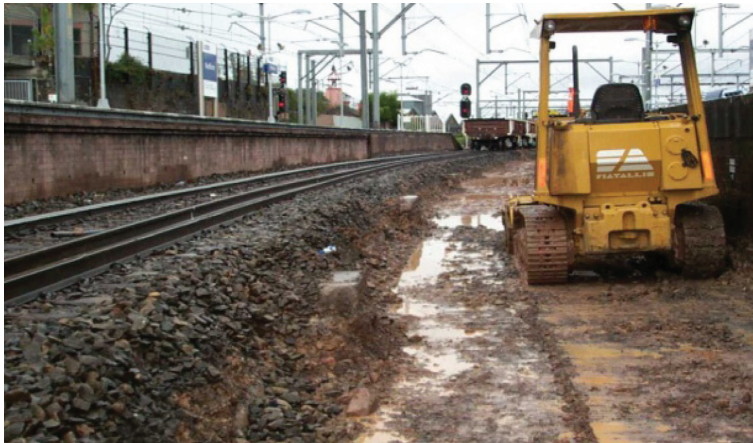
Figure 1.5 Insufficient drainage along a railway line in New South Wales, Australia.
