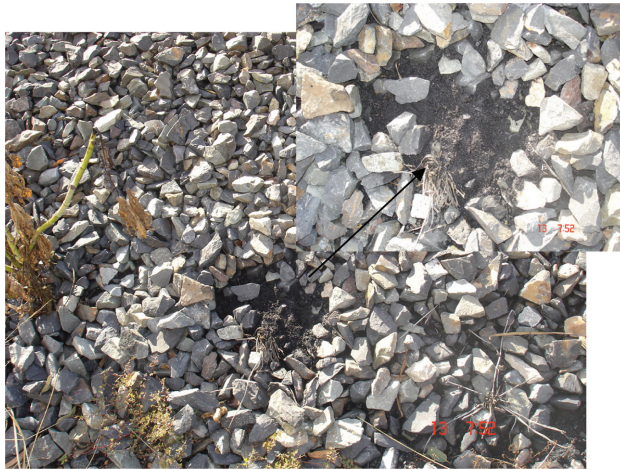
Figure C7 Intrusion of coal fines in to the shoulder ballast in a track near Rockhampton, Queensland.
