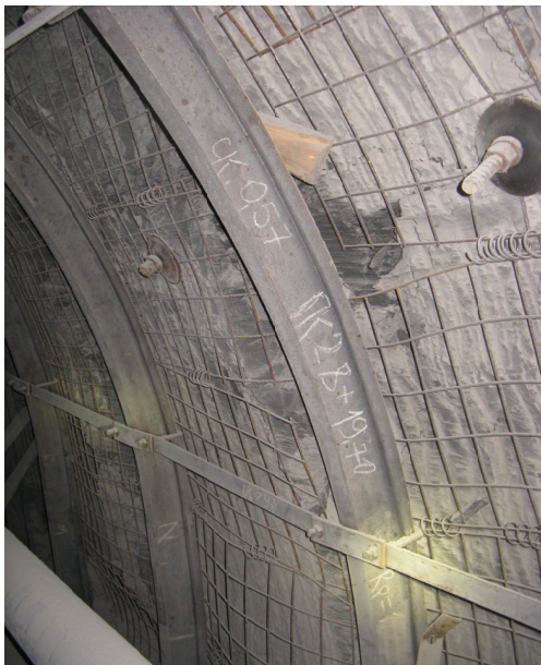
Figure 3. General view of “Ubileinaya” mine’s joining #2, supported by PFHS-15 made of SVP-19 profile in combination with rock bolt support in the roof of mine working.
