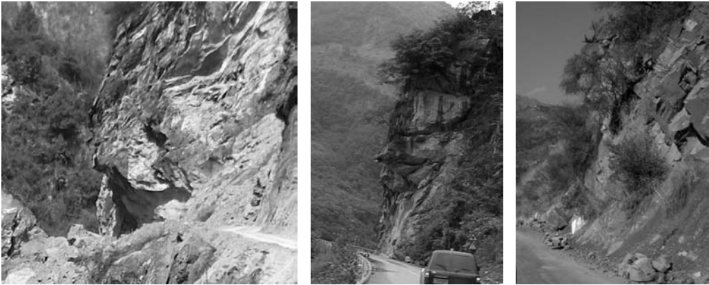
Figure 15.66 Rock falls from overhanging slopes or half tunnels.
