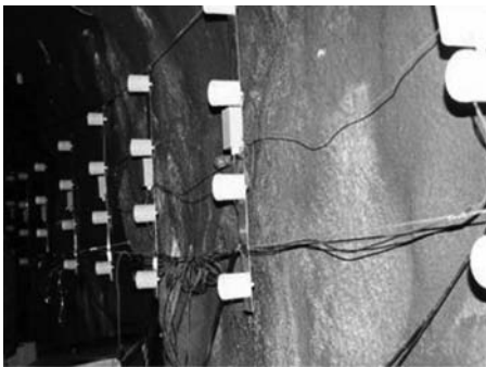
Light fixtures in slot tunnel after Test #4b
