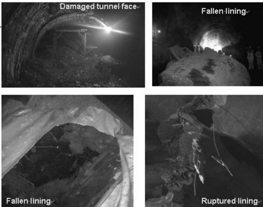
Figure 15.63 Earthquake damage at Jiujiaya Tunnel due to permanent deformations.
