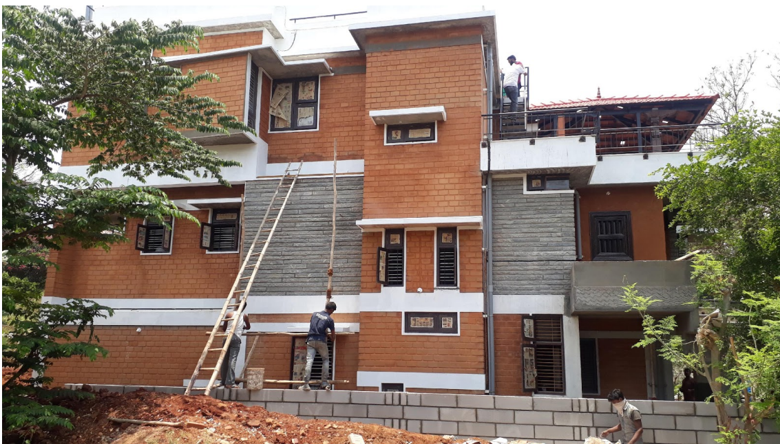
Figure 2: One of the thousands of houses using CSEBs in Bengaluru, under construction in 2019. Image Courtesy: Deepak Godhi ( www.thelivingstudio.in )
